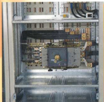
630 A functional unit
